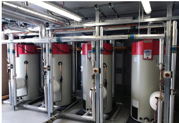
Gas-fired boilers and water heaters are tried and tested and still have a tremendous amount to offer
