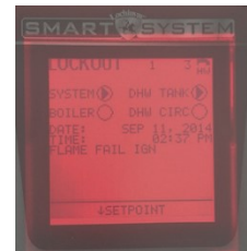
Boiler is not working
