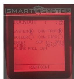
Boiler is not working
