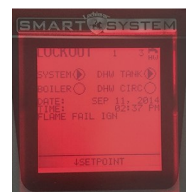
Boiler is not working
