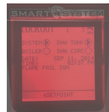
Boiler is not working
