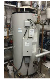
Typical pre-2019 installation
