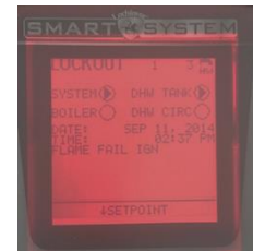
Water Heater is not working
