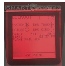
Water heater Locked out
